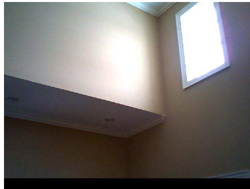
Side wall in entry way. 59.8 degrees in the dark area.
