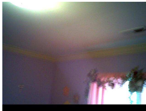
Daughters room left rear corner ceiling.
