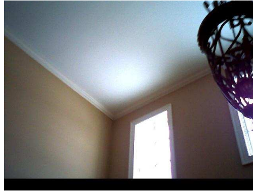
Ceiling in entry way. Insulation may be disturbed or not completely in place.
