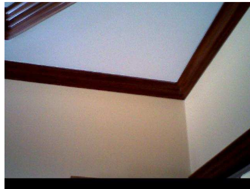
Main office looking back at entry door. Wall to the right over cabinets. Evidence of possible air infiltration or disturbed insulation.
