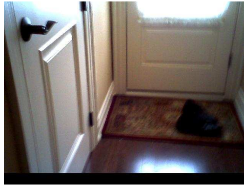
Side entrance door weather stripping gap.
