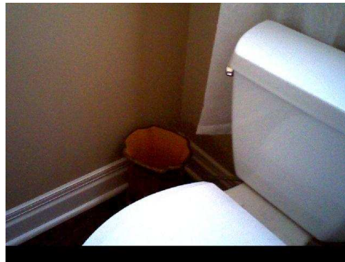
Bath in side entrance hall way. Left of toilet at baseboard.
