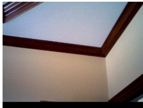
Main office looking back at entry door. Wall to the right over cabinets. Not terrible but evidence of possible air infiltration
